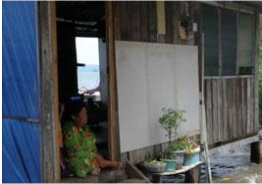
9 Families that live in the tidal swamps contend with deterioration of their homes. Volunteers helped put in a secure new foundation, repaired holes in the floor and put up a new wall (seen here).
